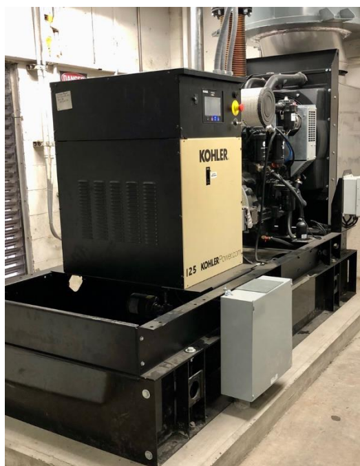
New Emergency Generator.
