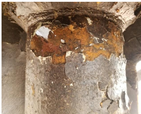
Old center column/RAS pipe.
