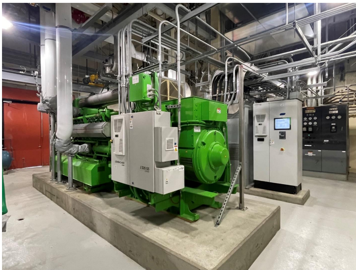
New cogeneration engine
